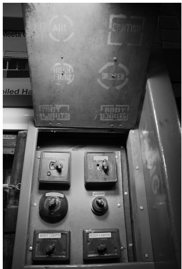
832n - Switch Cabinet
