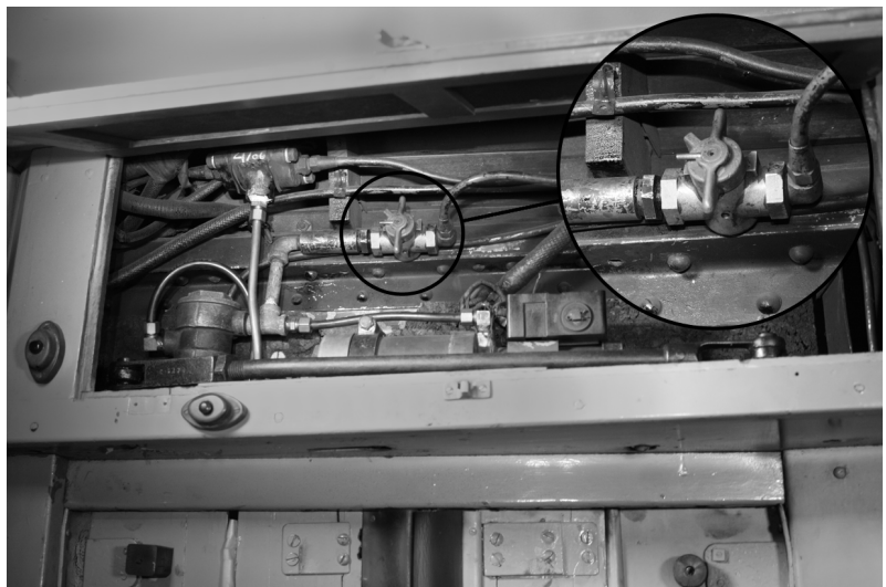
78 - Door Balancing Valve in the “balanced” position
