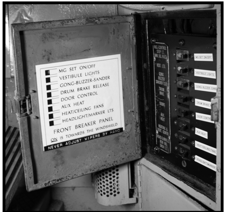
1711 - Front Breaker Panel
