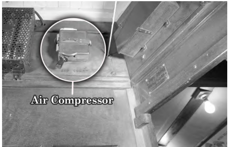
66 - Air Compressor Switch
