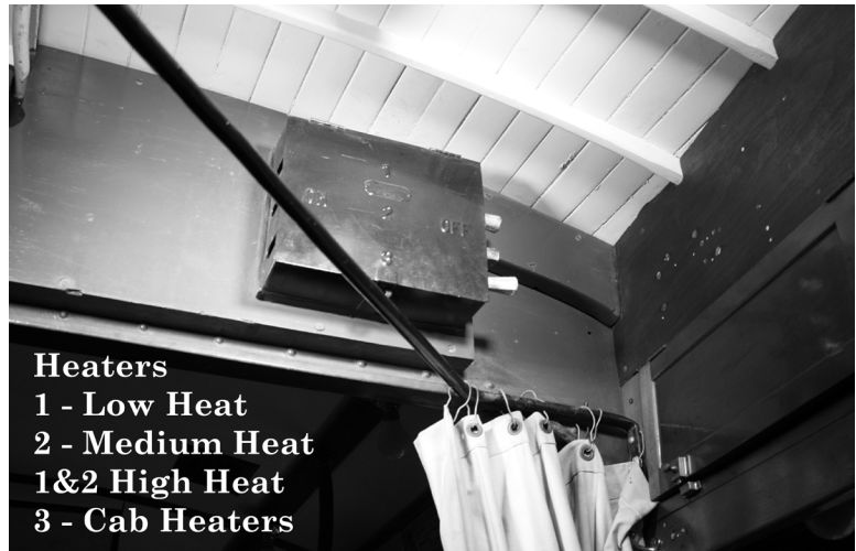
5326 - Heater Switch Box
