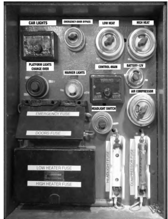
832w - #1 End Switch Cabinet
